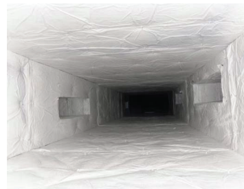
Image 2 - AHU4.1 Ductwork After
