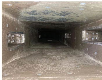
Image 1 - AHU4.1 Ductwork Before
